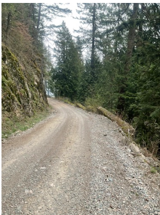
Woods approach, clean rock fall
