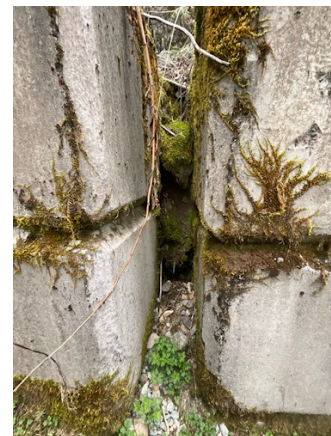
Geotextile visible in gap
