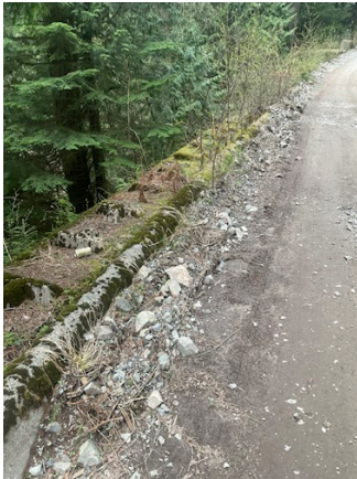
Barrier needs to be re established
